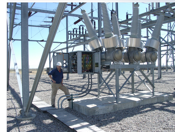
INL operates its own electrical power transmission and distribution system, which is linked with state-of-the-art SCADA, communications and cyber testing capabilities.
